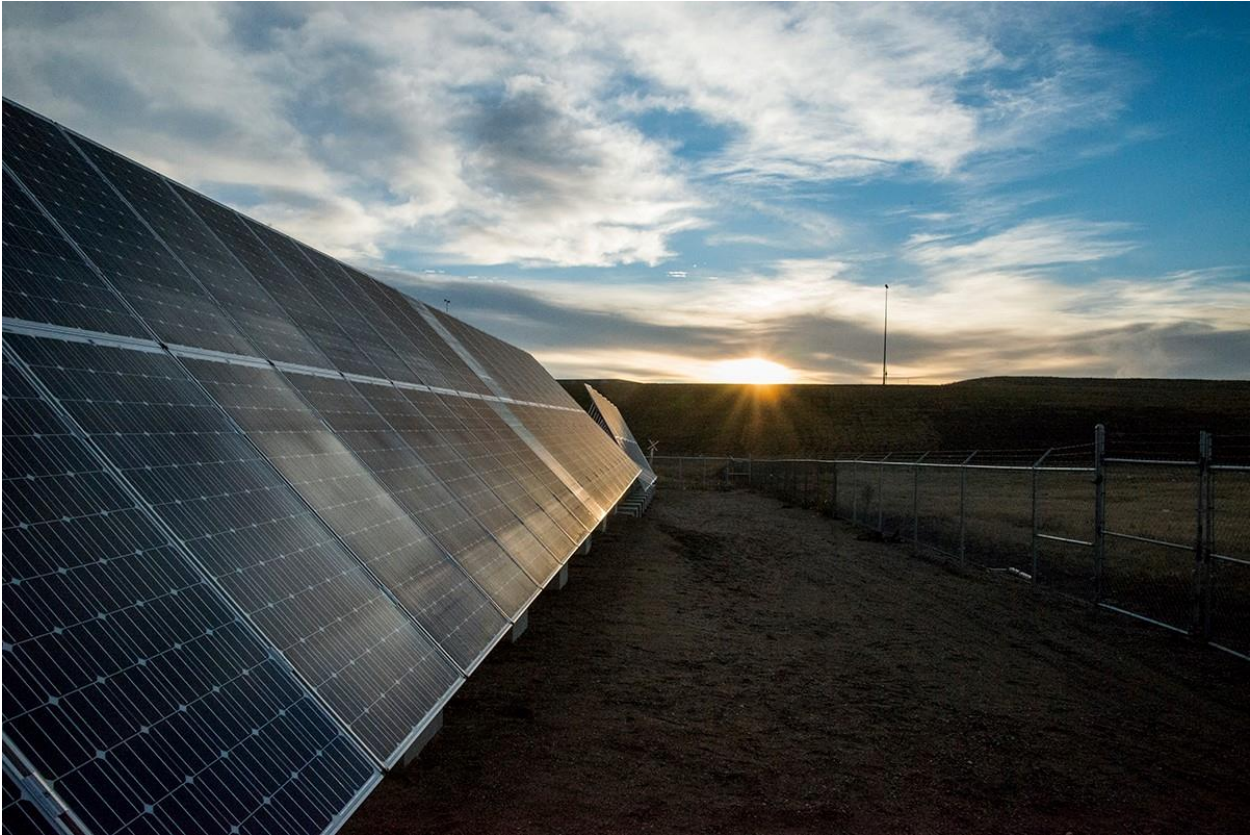
[Attached: City of Saskatoon and SES Solar Co-operative Solar Demonstration Site Photo Credit: Dale Read]
